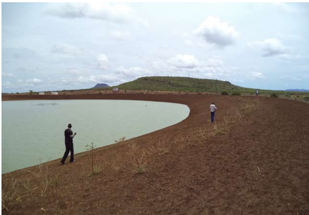
Figure 11. A Water barrier at Nakuromai, Eastern Equatoria State—the embankment is exposed to erosion
