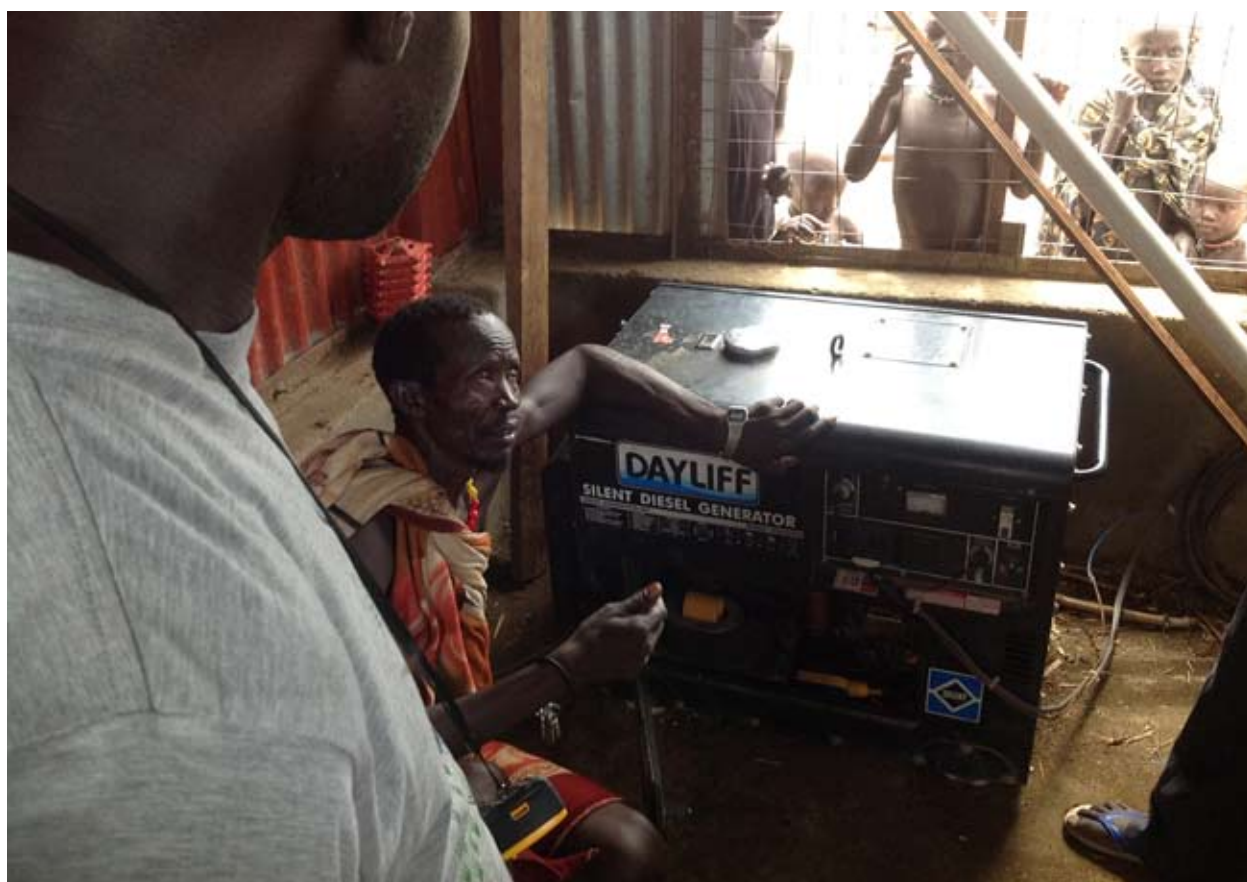
Figure 3. A defunct diesel generator intended to power the water at Lokoges, Eastern Equatoria State
