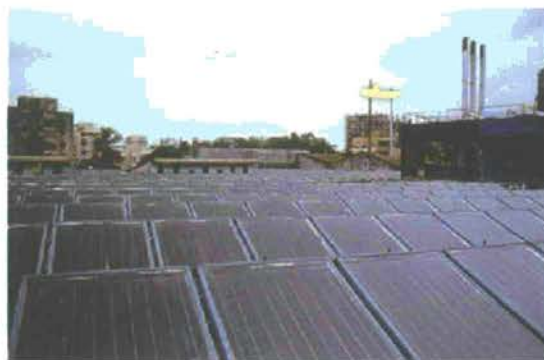
Photo 2.5 Solar power generation
