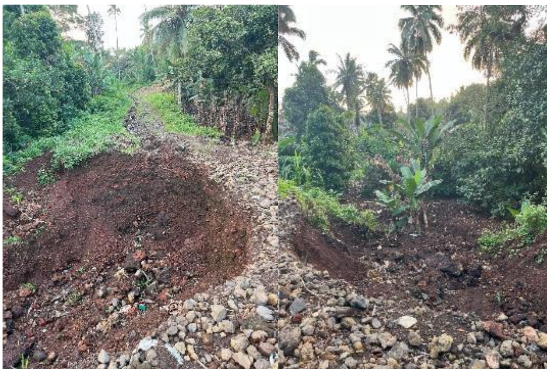
Figure 13 : Landslide and mudflow in Mjoyezi, Grande Comore (source: Baastel)
