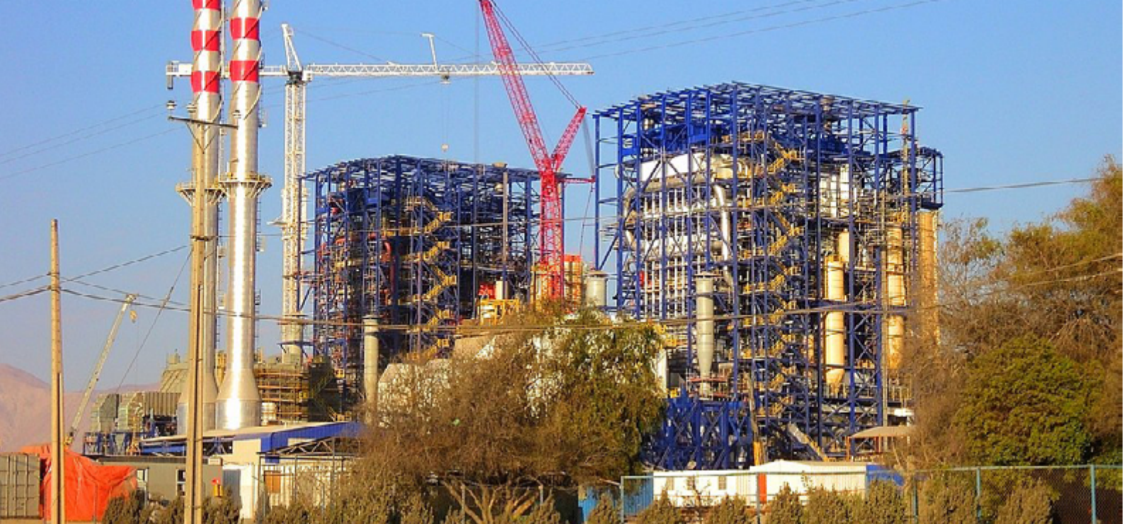
Thermal power generation infrastructure in Mejillones, Chile—illustrative of the generation assets addressed under Chile's power-sector decarbonisation pathway, including coal phase-down and closures. Photo: Victorodd. Wikimedia Commons.
