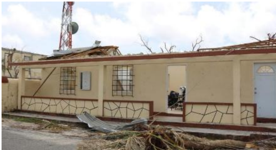
Figure 3. Office buildings in Barbuda left with no roof, destroying equipment and IT systems after the passage of Category 5+ Hurricane Irma in September 2017
