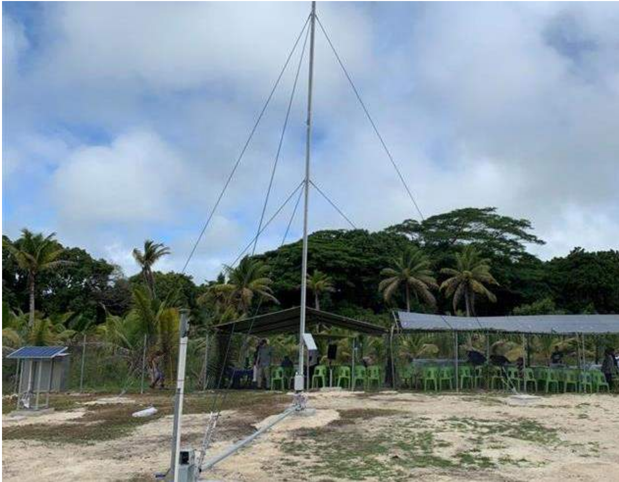
Automated Weather Station in Niue, Pacific Programme
