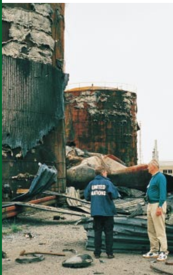
Inspection of damaged oil tanks
