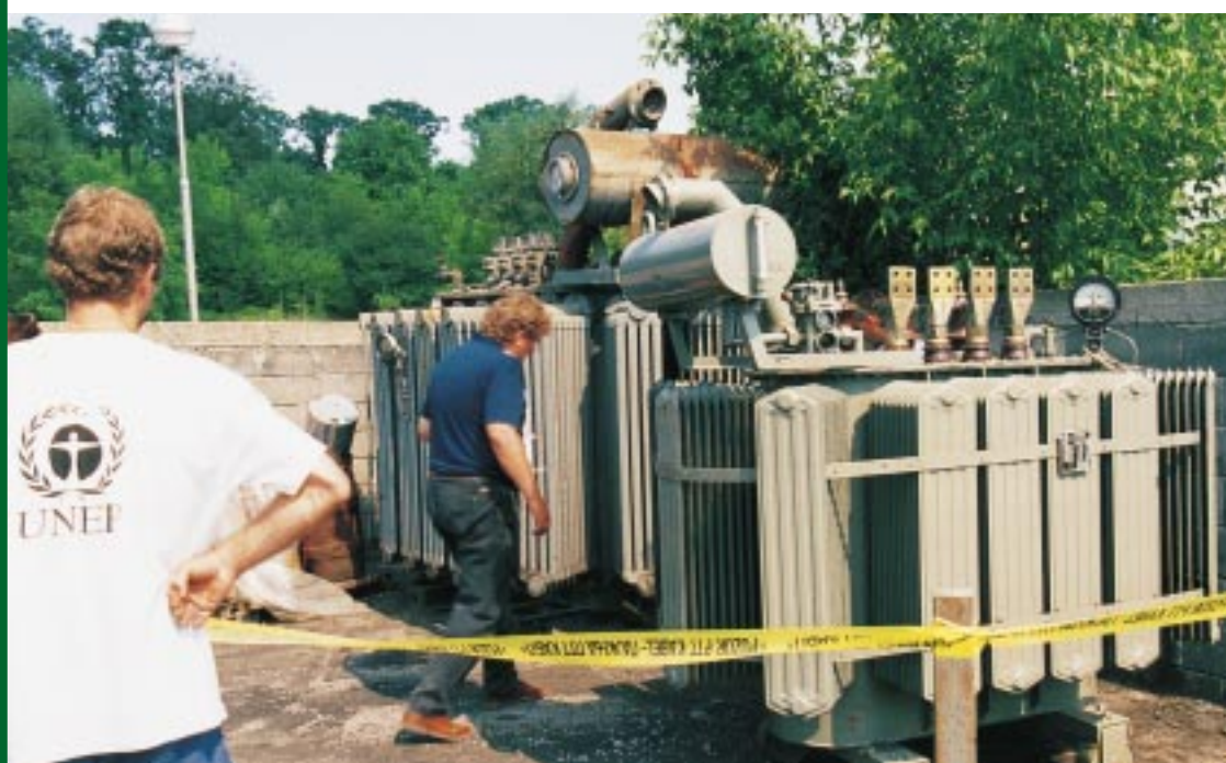
Inspection of damaged transformers
