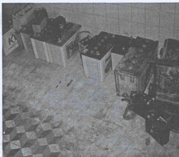
Pic.2.12: The spillage of acid during recharging process and its negative effects
