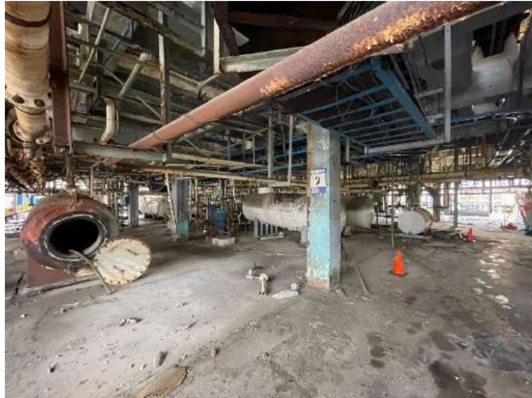
Figure 2. View of the interior of the plant in Monterrey
