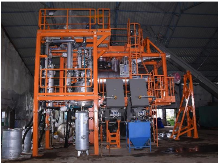
Condensation unit and clean soil discharge
