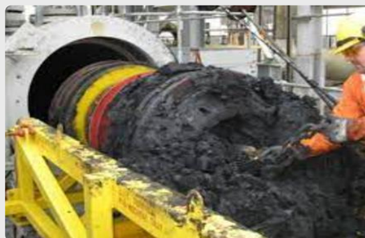
Figure: Sludges obtained during pipeline “pigging” operations
