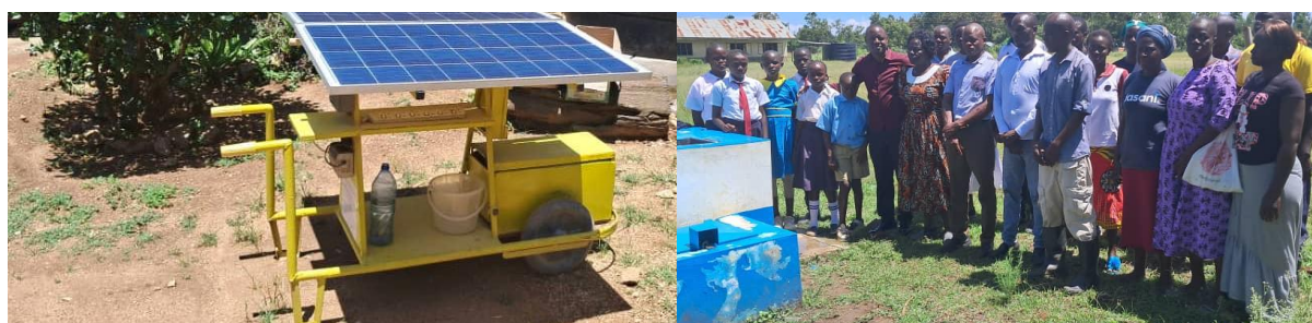
Figure 8: Portable Solar powered water pumping system (left) and Borehole supported with solar system at Kahoya Primary School in Kenya (right).
