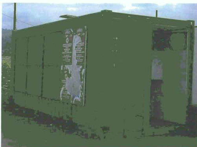
Figure 1. Don't judge a telephone container by its exterior...
