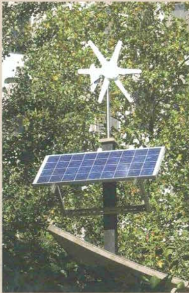
Renewables at a Primary School in Kings Cross, London. As well as lighting play structures in winter evenings, the installation forms part of teaching activities.
