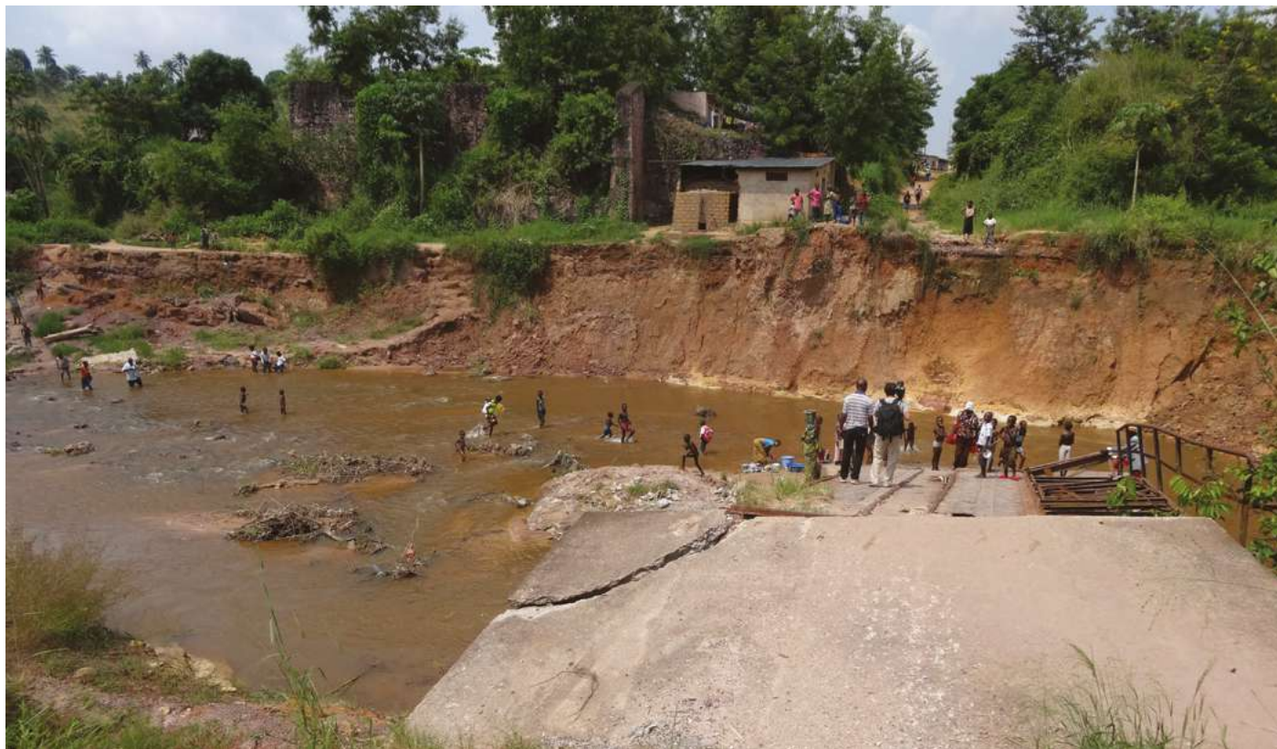
Bridge damaged by 2012 flooding in Kasangulu
