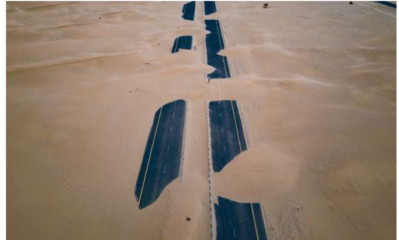
Road after a sandstorm in Dubai (Schwaerzler 2017).
