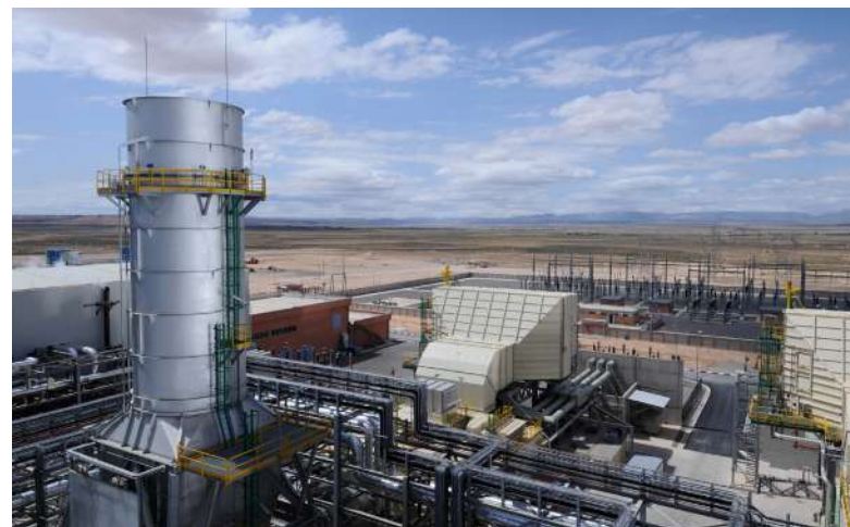
Thermo-solar power plant in Morocco (World Bank 2010)
