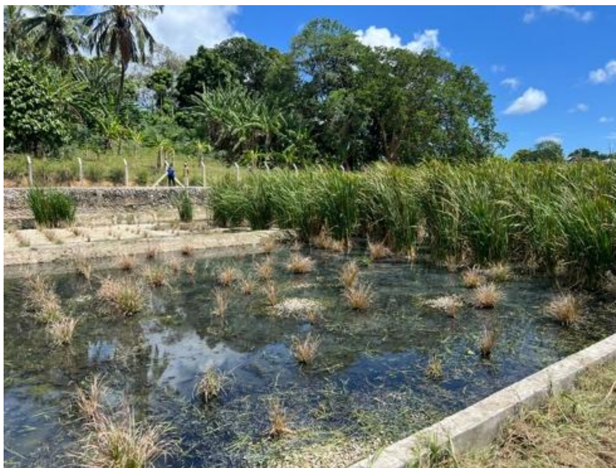
Figure 12: Msingini Wastewater treatment facility in Chake Chake town, Pemba
