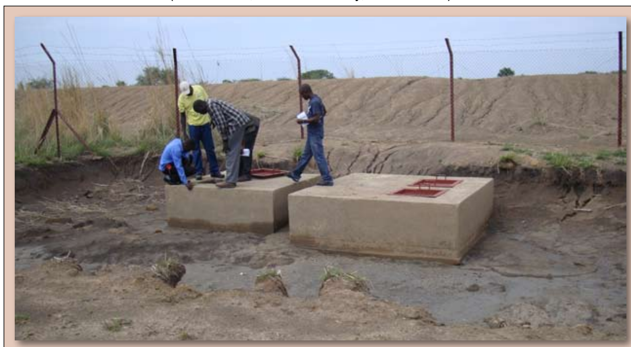
Figure 10. Inlet box constructed above the flood level resulting in haffirs being unable to receive runoff (Abiriu Haffir, Cueibet County, Lakes State)
