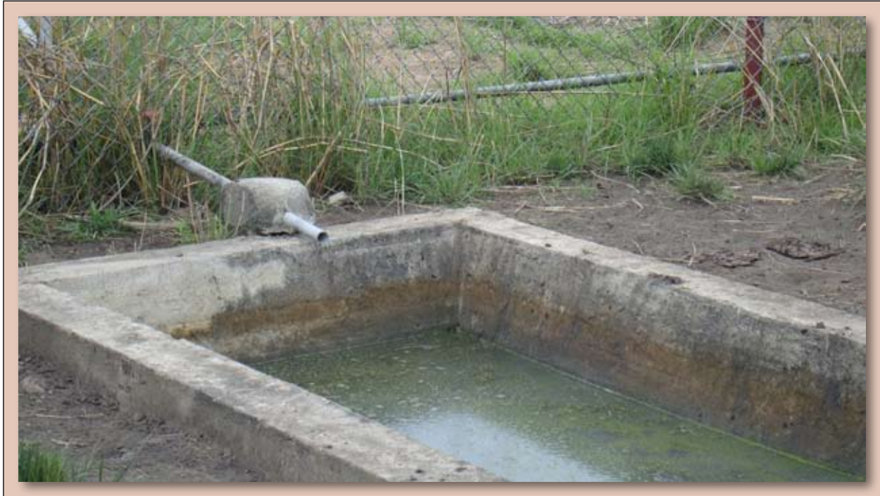
Figure 15. Small size pipelines installed as inlets for cattle troughs that can cause unnecessary queuing at haffir sites (Nyangkot Haffir , Rumbek Centre County, Lakes State)
