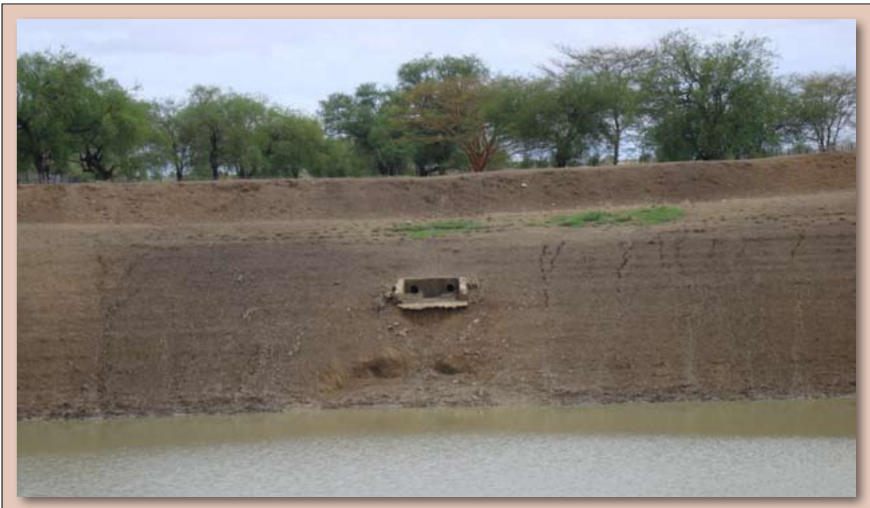
Figure 8. Outlet of inlet structure without energy dissipation provision (Lokoges haffir , Kapoeta North County, Eastern Equatoria State)
