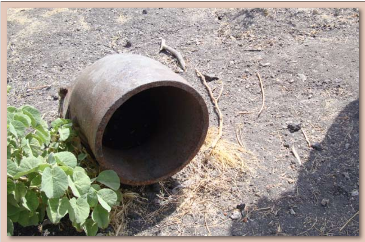
Figure 11. Inlet pipe constructed above the flood level resulting in haffirs being unable to receive runoff (Oriny Haffir, Fashoda County, Upper Nile State)
