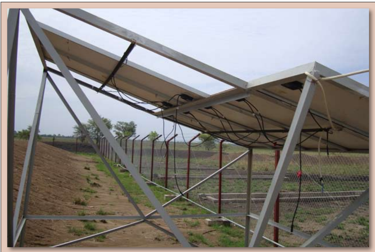
Figure 12. Blown up solar panels (Abiriu Haffir, Lakes State)
