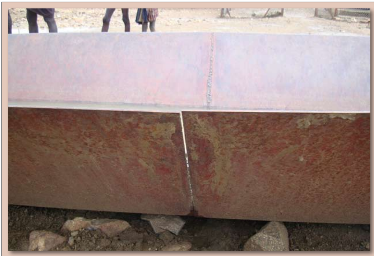
Figure 14. Poorly welded cattle troughs (Abiriu Haffir , Lakes State)
