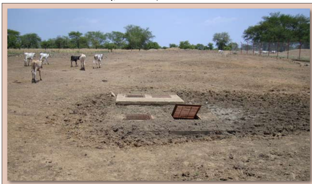
Figure 6. Inlet boxes filled with sediment material (Nyangkot haffir , Rumbek Centre County, Lakes State)
