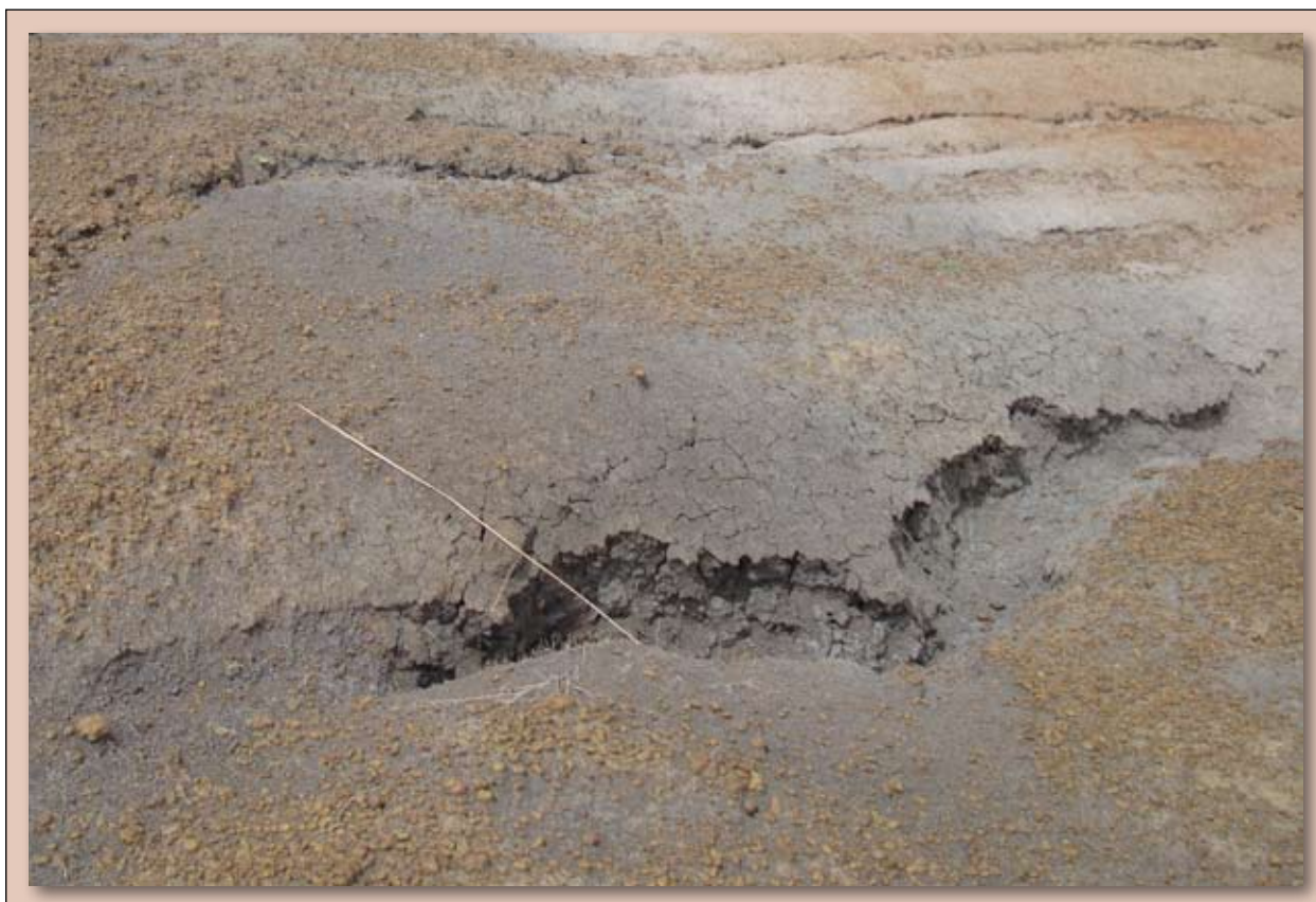
Figure 13. Poorly compacted wall of a reservoir (Lokoges Haffir , Eastern Equatoria State)
