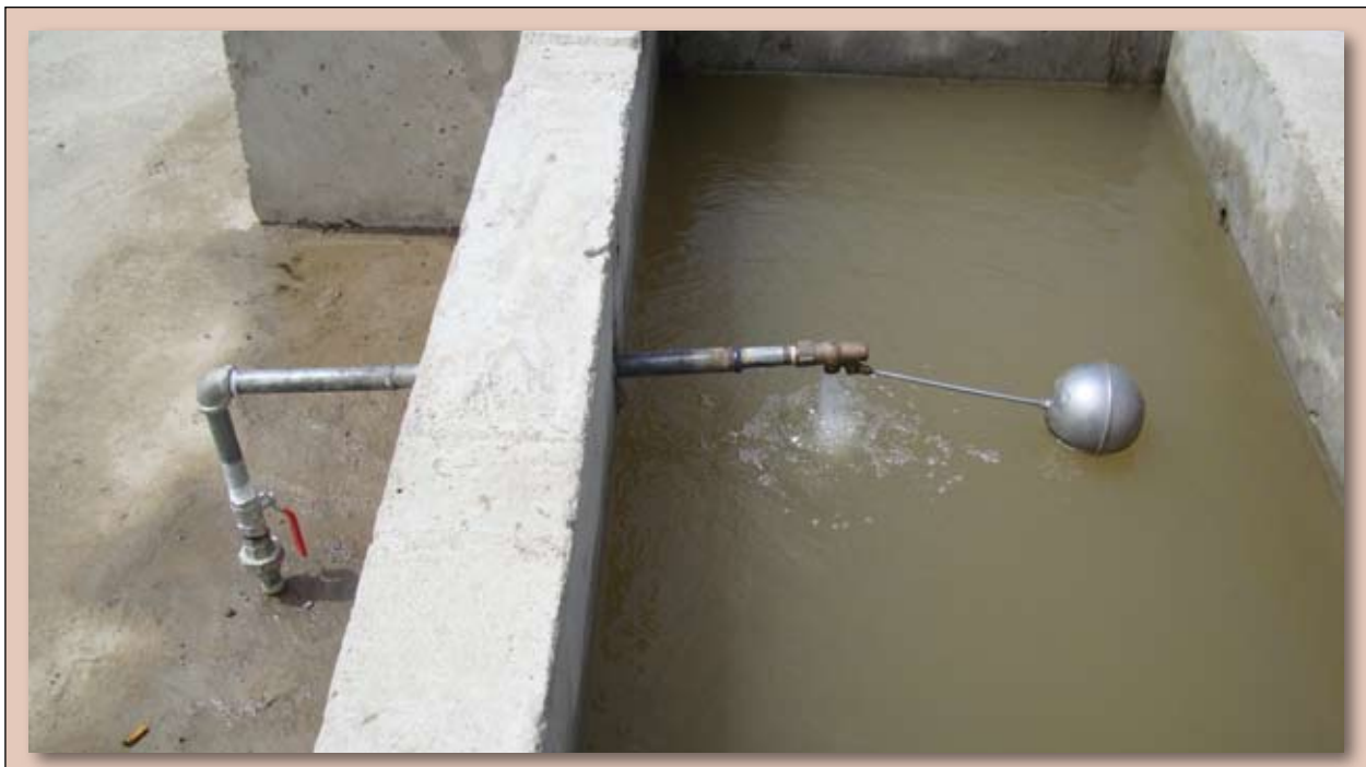
Figure 15. Small size pipelines installed as inlets for cattle troughs that can cause unnecessary queuing at haffir sites (Pul Dol Haffir , Uror County, Jonglei State)
