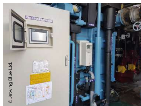
The vapour absorption chiller at Jetwing Blue
