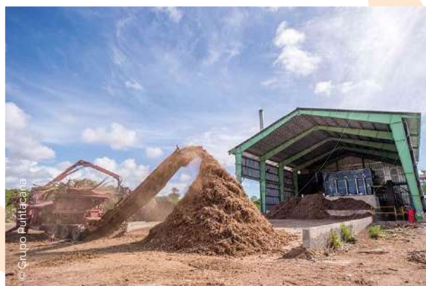
Biomass boiler, at Punta Cana Laundry Service.
